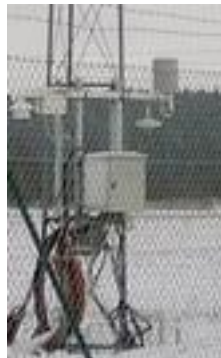
Compact fan-ventilated solar shelter
